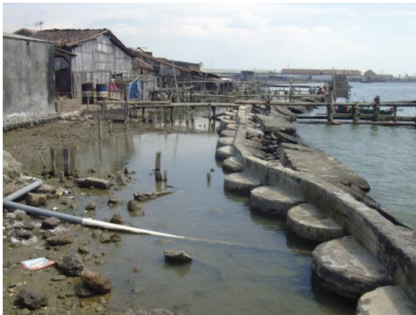
Fig. 19. Damaged infrastructure due to erosion and abrasion.
