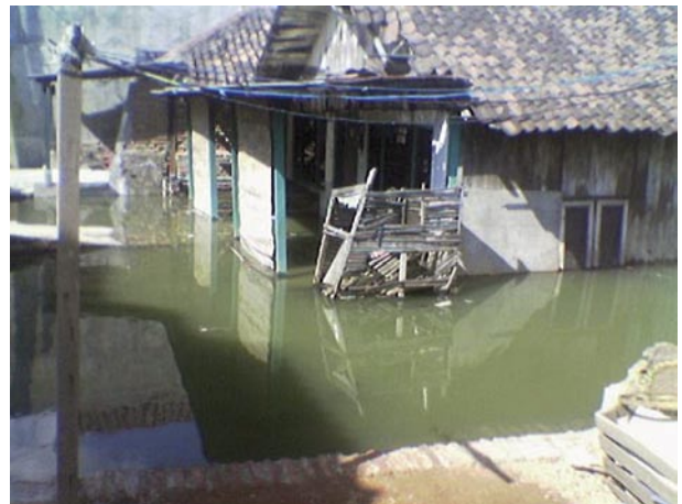
Fig. 10. House damage due to tidal inundation.
