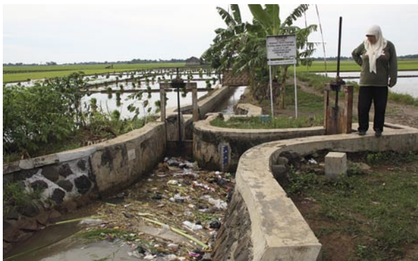
Fig. 13. Garbage and waste disposal in channel.
